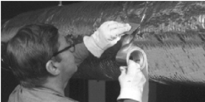
Fig. 11. Sheet metal duct with fibrous glass wrap.
