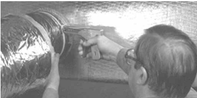
Fig. 17. Insulated flexible duct.
