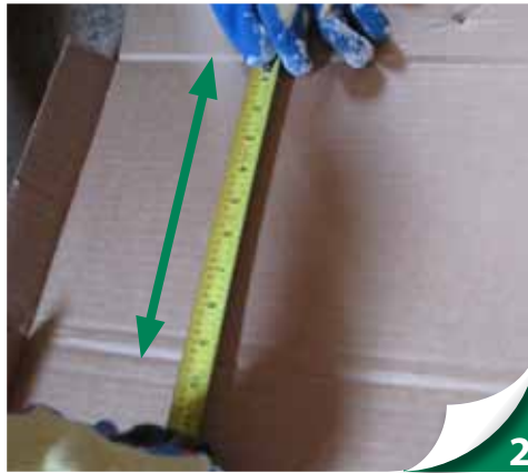
Measure and mark the height on the baffle. Verify the height allows for 1-inch of required air space.
