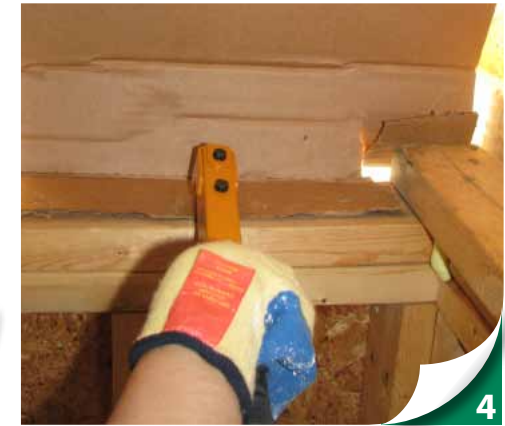
For all eaves with vents, fasten soffit dam material to the attic framing or permanent blocking so that insulation will completely cover the top plate.
