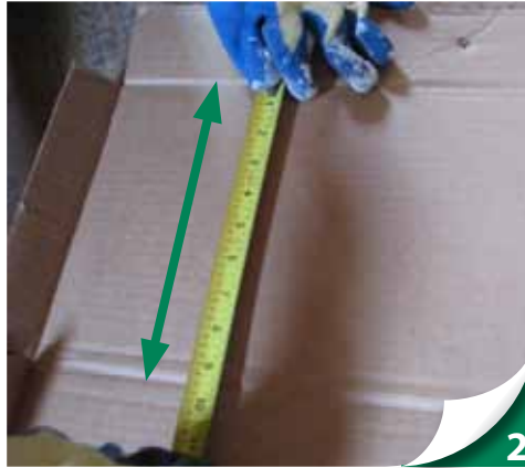
Measure and mark the height on the baffle. Verify the height allows for 1-inch of required air space.
